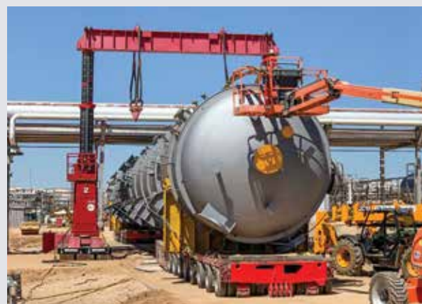
FIG. 1. The installation of three large pressure vessels at a refinery in the Texas panhandle required minimal disruption to the plant's six-figure throughput, while taking up as little space as possible.
