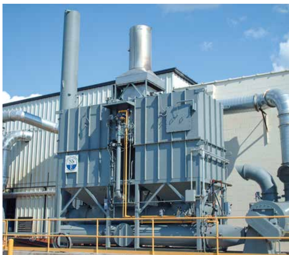
FIG. 2. A regenerative thermal oxidizer employs ceramic media to capture heat from oxidation to reach thermal efficiencies of up to 98%.
